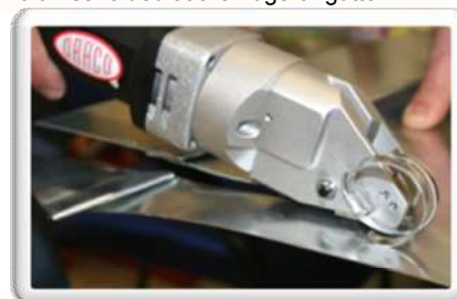
cutting through double lock seam 6 times folded at the ridge or gutter
